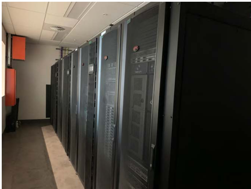
The new server room
